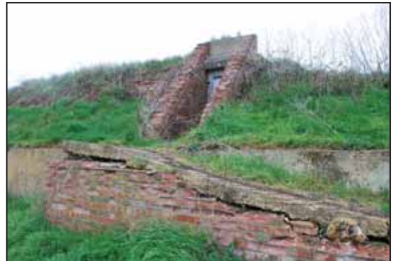
Tending to this neglected blast pen will form part of the work to be carried out by the Kenley Revival Project.
